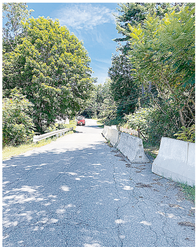
Project funds will be used to replace bridges at Mountain Home Park in West Brattleboro.
