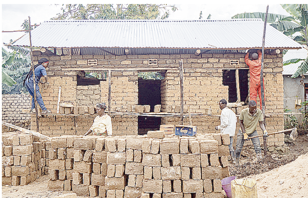
It costs just $3,000 to build an Inshuti home in Rwanda, including all building material, labor, project coordination, and home provisions.
