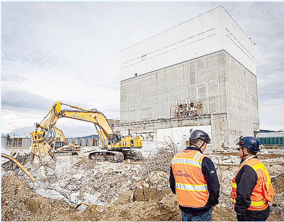
The deconstruction of the former Vermont Yankee nuclear power plant in Vernon continues. The reactor containment building on the right, seen here during a media tour on Oct. 10, is empty and is the last large structure on the site.
